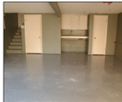
Transformation: Here's the end result after the floor was cleaned with a pressure washer and coated with Thompson's Water Seal Garage Floor Epoxy Coating.
