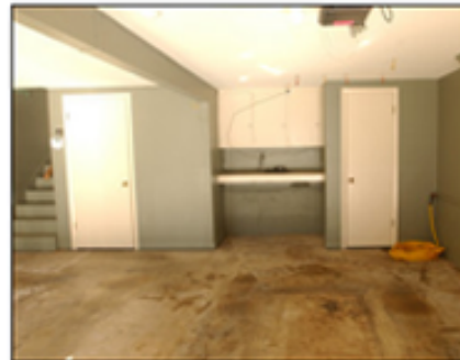
Major mess: It would take hours to clean this garage floor by hand. Photo courtesy of Thompson's Water Seal.
